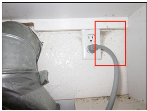
3.1 Picture 1 view above microwave
