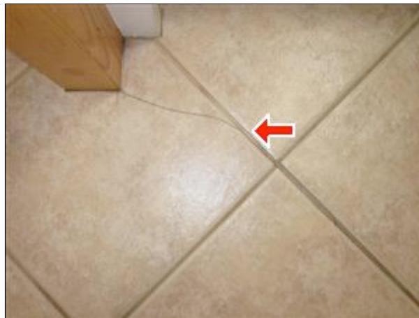
3.2 Picture 2 cracked tile
